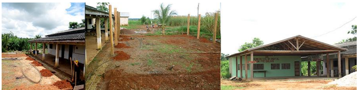
Figure 6. The building of a community center in what had been the main house of a ranching state. Left and Center: the 2011 construction project. Right: the new common area in operation in 2012.
